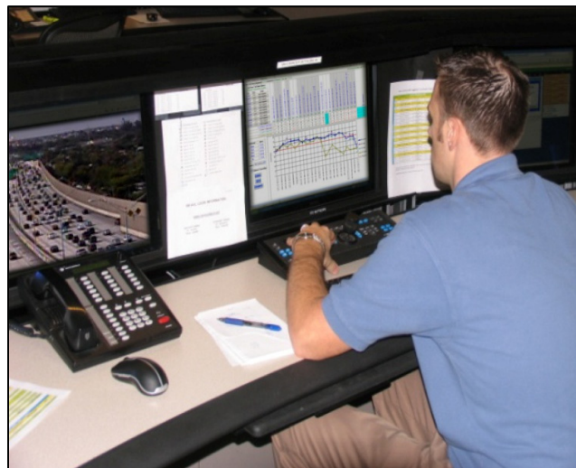
Express Lanes Operator monitors and manages 95 Express with CCTV cameras and the Express Lane Watcher software.
